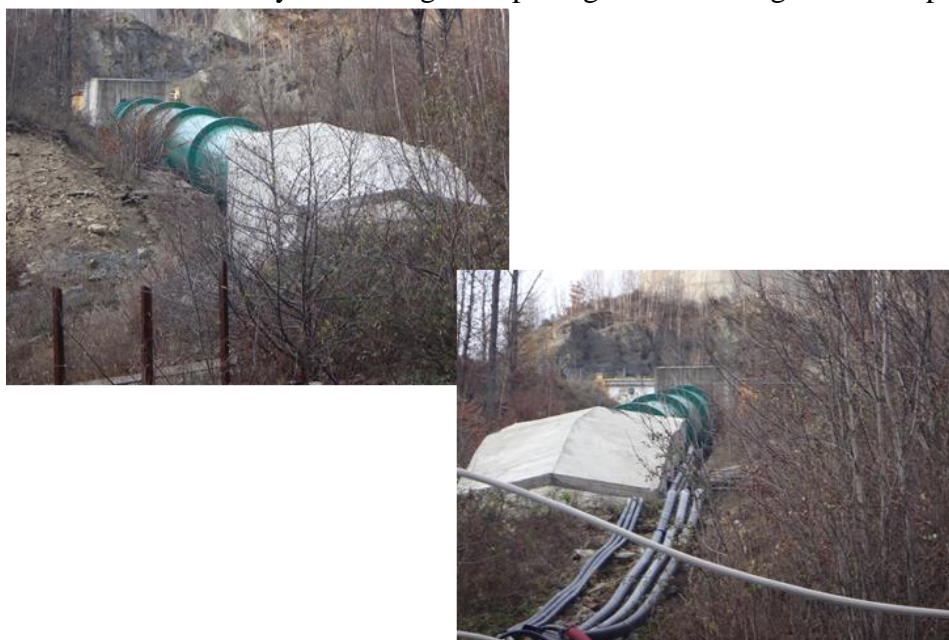
Fig. 13 The penstock from the power structure of CHE Dumitra
